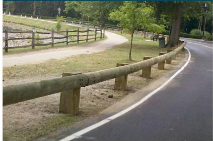
Guardrails (Salt Point)
